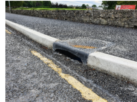
SIDE ENTRY GULLY
