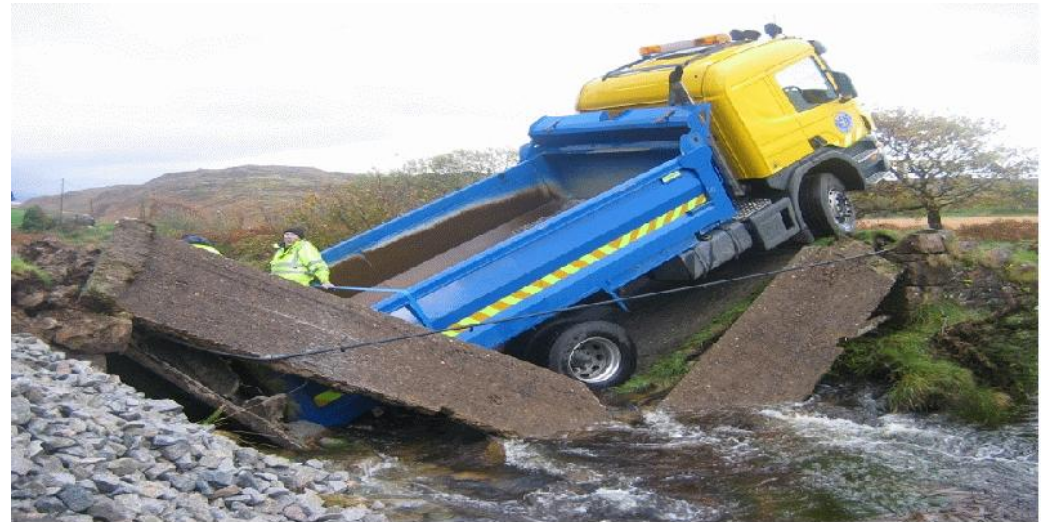
Rare example of failure under load
