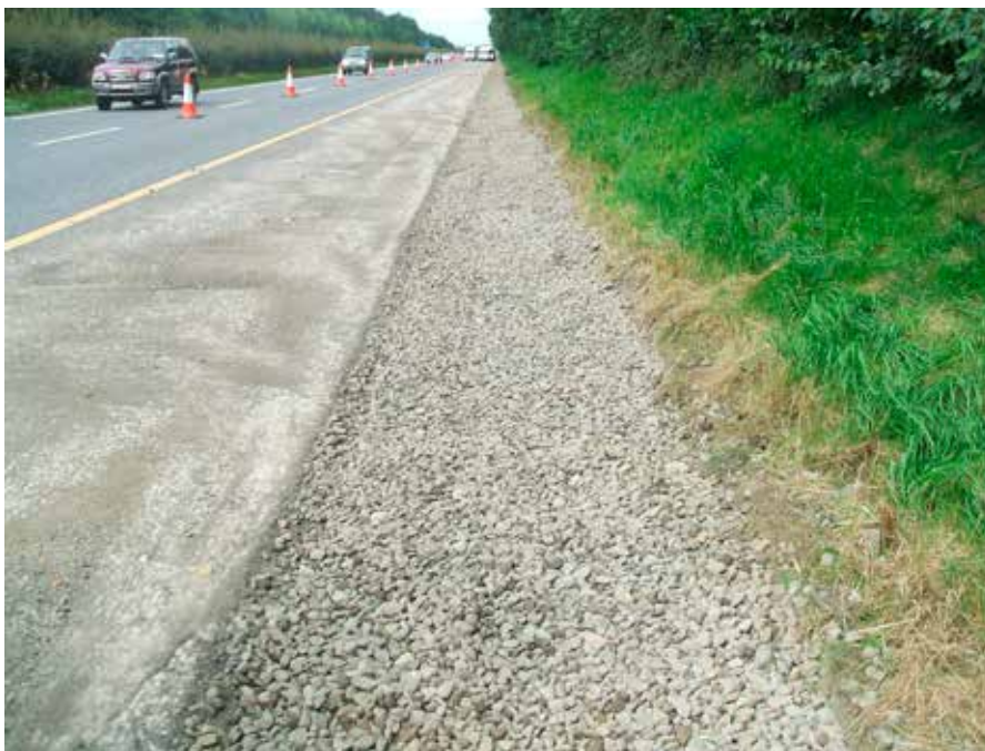
Plate 18 Regenerated French Drain. After clogging the combined filter drain can be cleaned.
