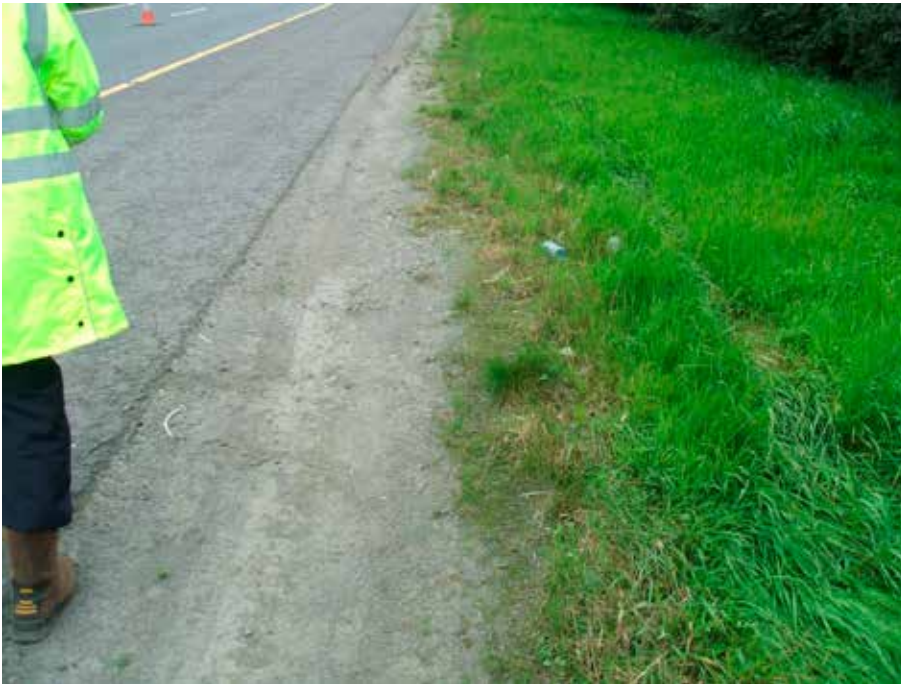
Plate 4 Clogged Filter Drain. Combined filter drains (French Drains) can become clogged with silt resulting in surface runoff bypassing the system and entering the receiving environment. In vulnerable areas groundwater can be a potential receptor.
