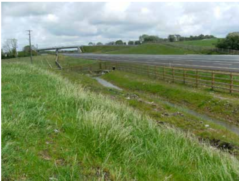
Plate 8 Lined conveyance channel linking carrier drain from motorway to a wetland. Channel is lined to protect an underlying karst aquifer of regional importance.
