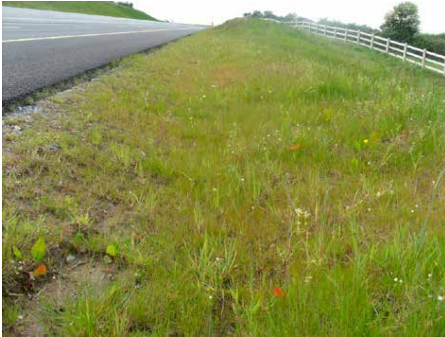
Plate 19 Grassed surface water channel used to treat and convey surface runoff. Contains a mix of grass types to attenuate flow.
