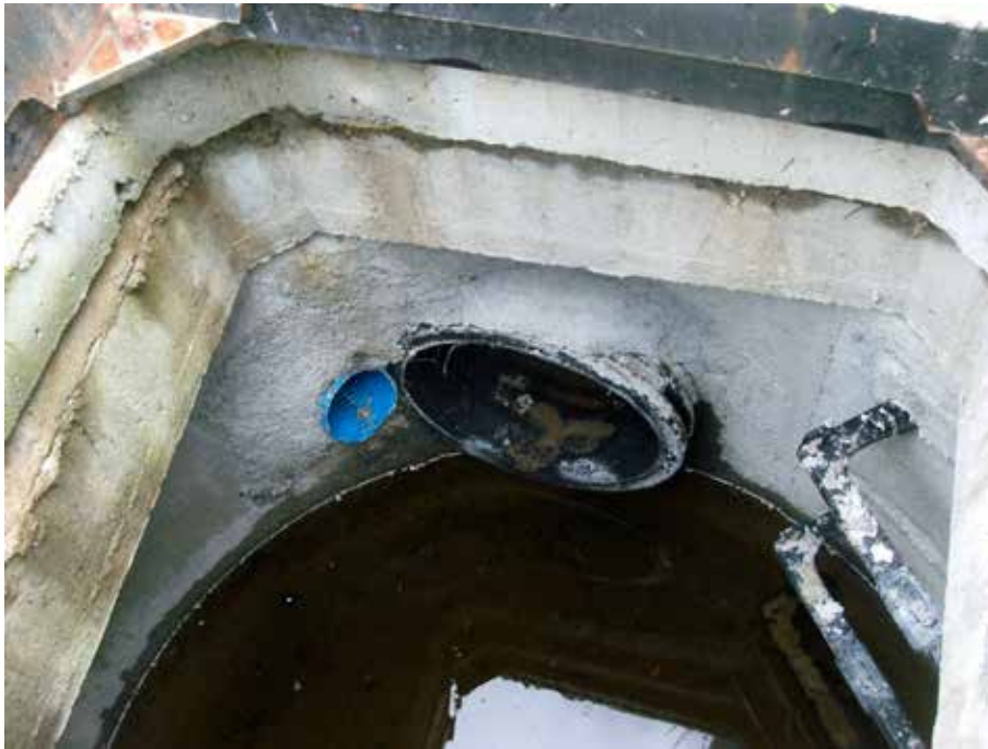
Plate 16 Catchpit with main carrier drain in black and slotted pipe from fin drain in blue. Surface water from road runoff and groundwater are mixed in the above catchpit.
