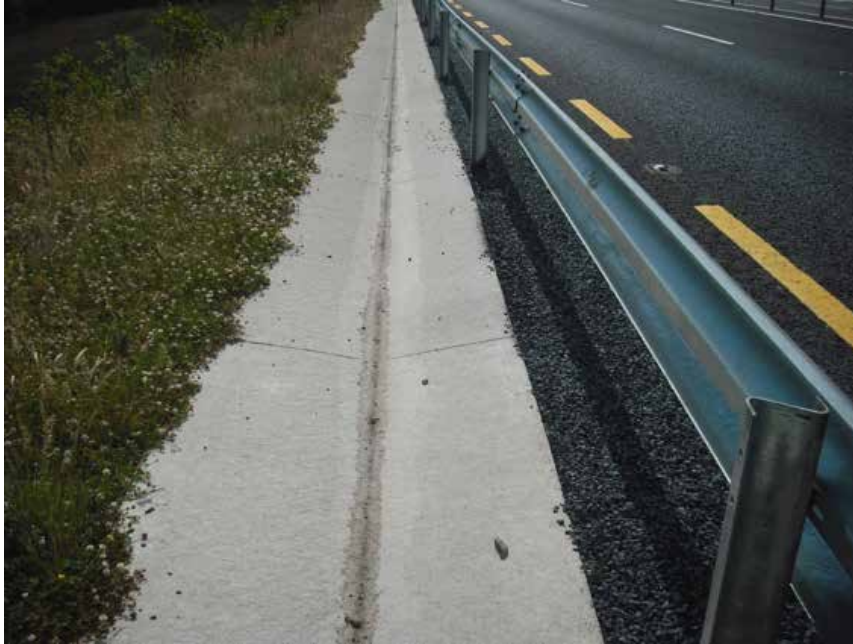
Plate 1 Concrete channel used to convey surface runoff, part of a sealed drainage system. A separate fin drain, below the concrete channel, is used for conveying groundwater.
