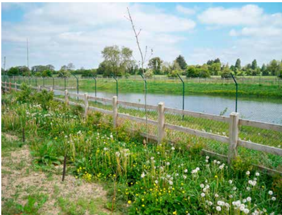
Plate 6 Detention Basin. Typical storm water attenuation system used on many National Road Projects.
