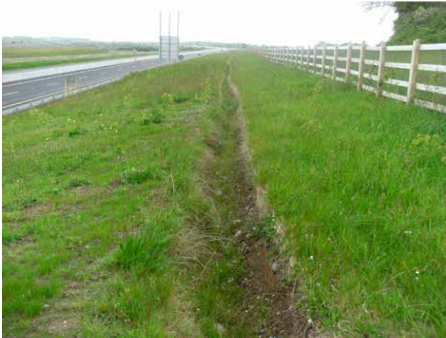
Plate 14 Interceptor ditch intercepting runoff from the natural catchment before it enters the road drainage system.
